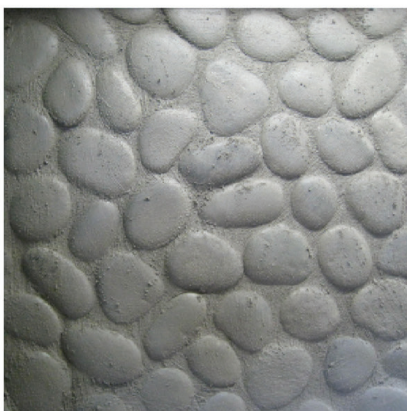
Grout is recessed
